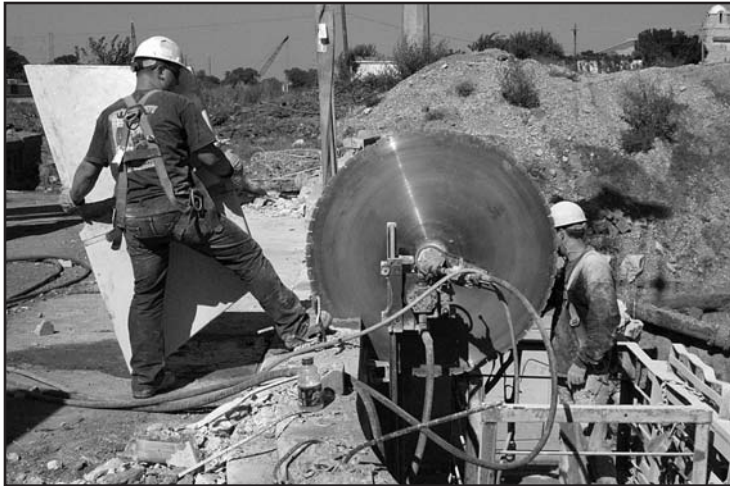
Two passes were made to cut the beam. This is the second and largest blade with the guard about to be installed.
