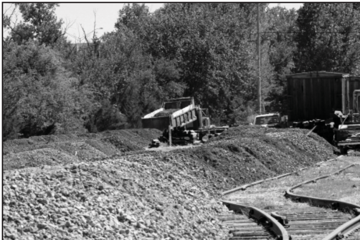
Across a field of ballast at Owanda siding a truck prepares to dump another load
